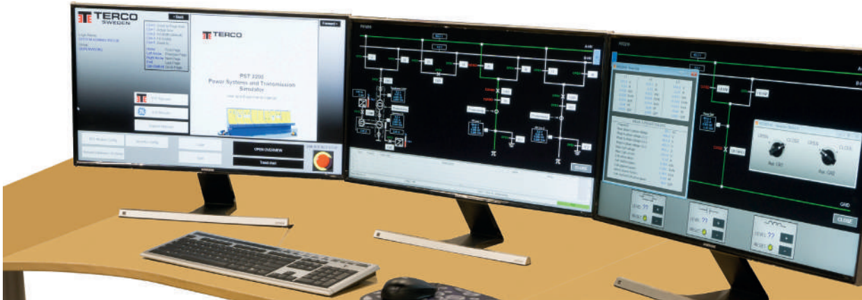
To provide the best possible overview the system is delivered with 3 screens
