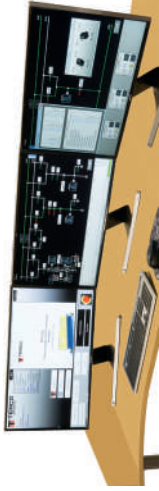
PST2250-15 SCADA System
